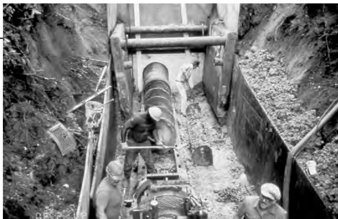
The Conservancy's jack-and-bore project placed a 90-foot section of steel pipe under M-24 so that cold bottom water from Lake Orion could flow into Paint Creek and allow trout to survive there.
